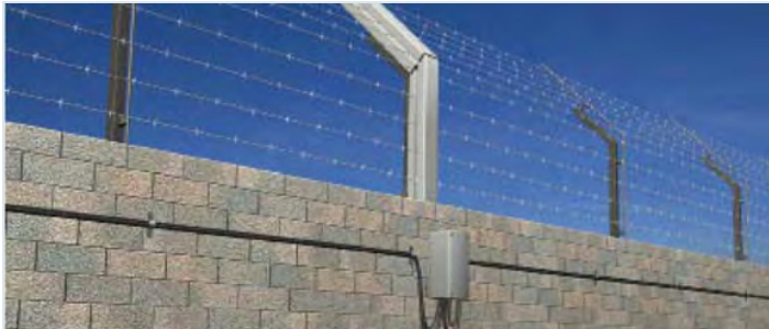
Wall-top installation with sensor post and processor housing
